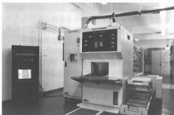
Photo 1 Contamination inspection monitor 12)
